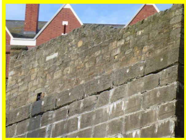
Gap between blockwork in upper section of wall (/4601C05)
