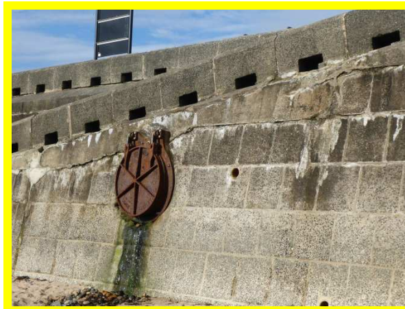
Previous repairs and local open joints which would benefit from maintenance (/4501C07)
