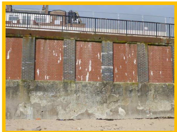
Abrasion damage to wall toe and cope (/4601C02)
