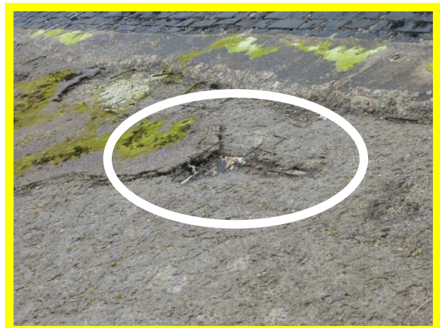
Exposed rebar (/4701C27)
