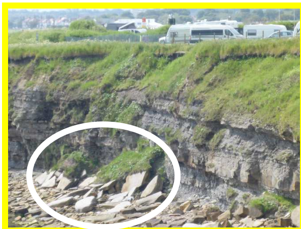
Rock falls in hard material along lower cliffs (/4401C22)
