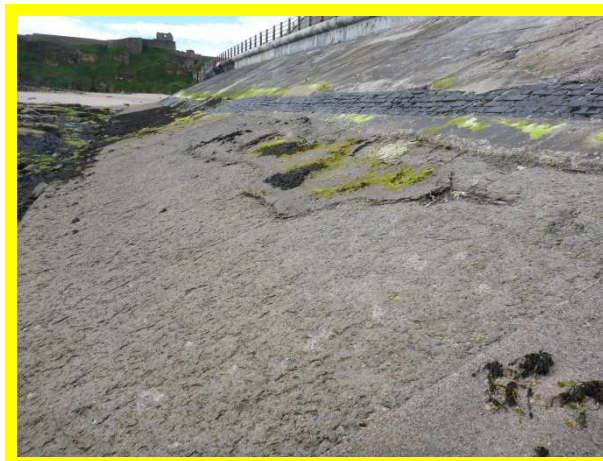
Sea wall in fair condition with abrasion of the apron leading to exposed rebar (/4701C27)
