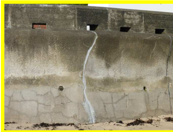
Previous repairs to rendered sea wall (/4501C08)
