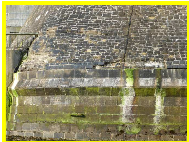
Two sections of missing brickwork (/4601C06)
