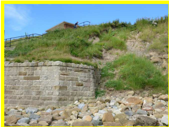
Slumping in cliffs near northern end of masonry wall (/4701C17)
