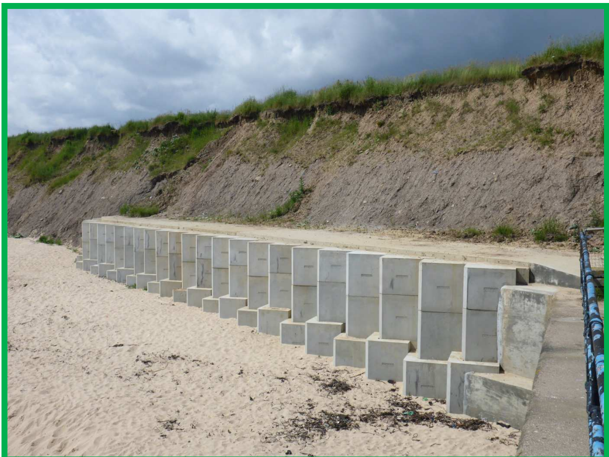
New T-Block units (constructed in 2014) prevent outflanking at the southern end of Trinity Road seawall (/4501C04)
