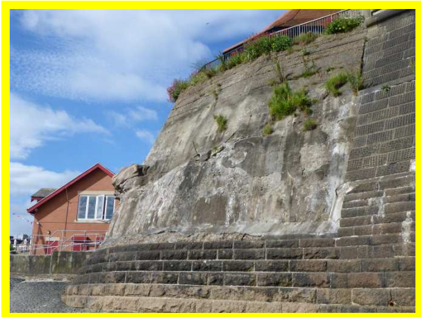
Final section of sea wall in generally fair condition, but with some defects at the tie-in requiring remedial attention (/4701C06)
