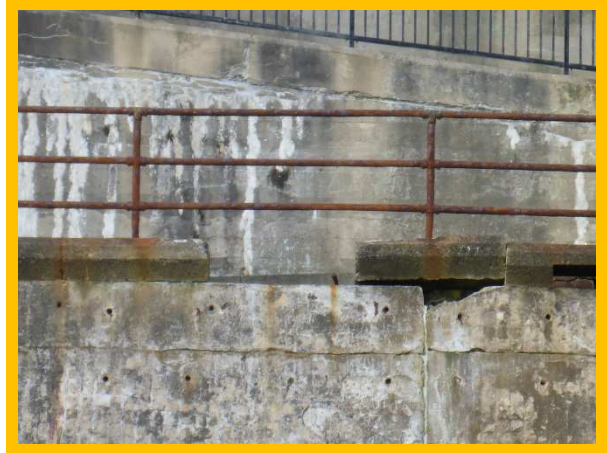
Missing section of cope (/4601C03)
