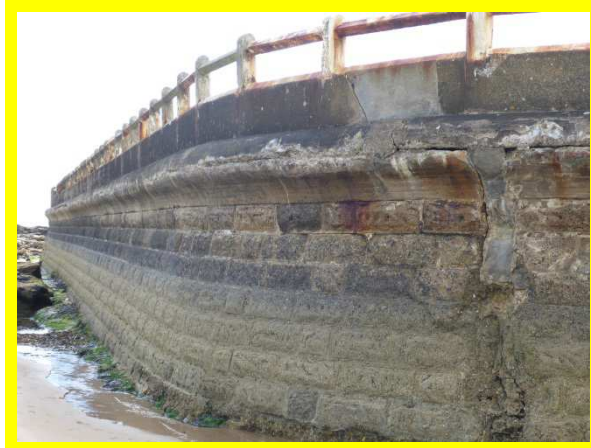
Further repairs to an area of previous repair at the Outdoor Pool (/4701C24)
