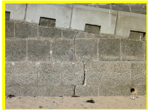
Cracked blocks in wing wall to access steps (/4501C07)
