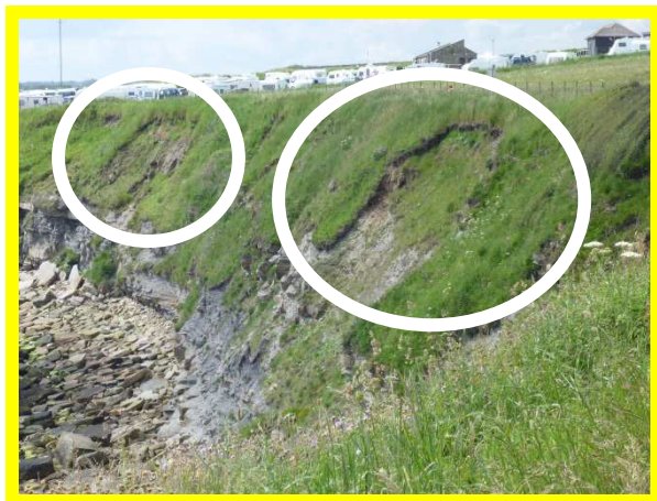
Slippages in soft material along upper cliffs (/4401C22)
