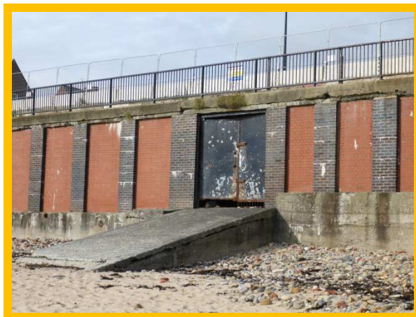
Cracking to boat ramp (/4601C02)
