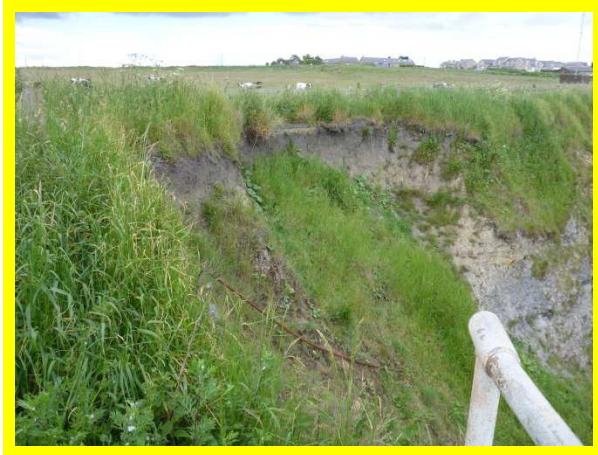
Slippages in soft material adjacent to Hartley Cove access steps (/4401C23)
