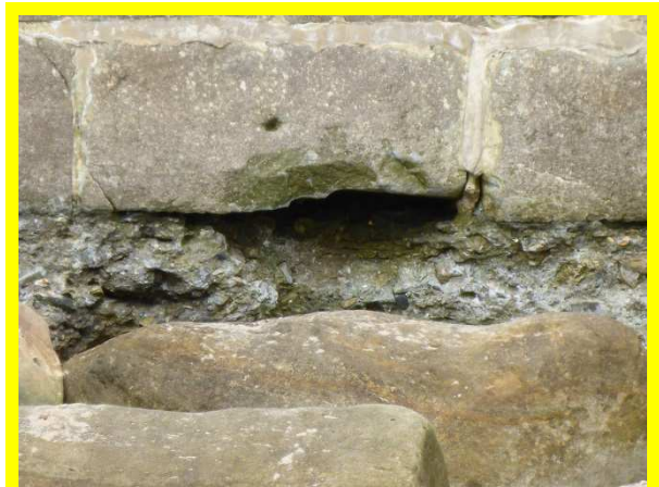
Undercutting at toe of wall (/4701C17)
