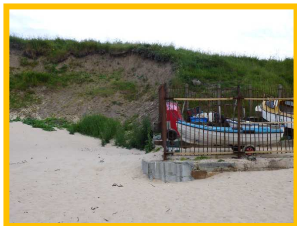
Erosion of the cliffs immediately south of the boatyard (/4501C05)
