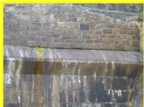
Gap between blockwork and masonry walls (/4601C04)
