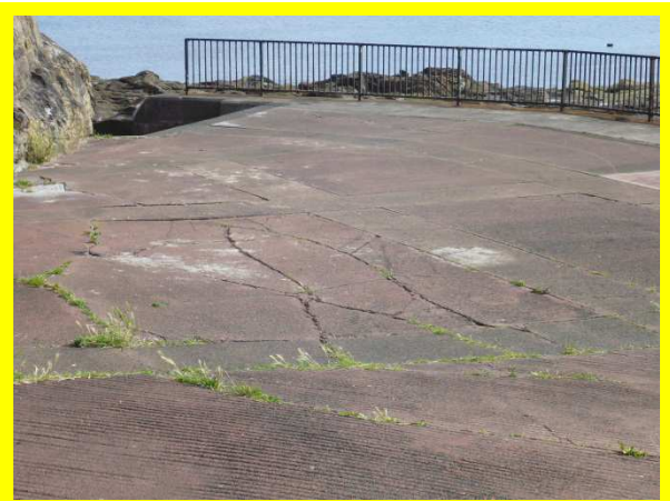
Cracked promenade deck at northern end (/4601C10)
