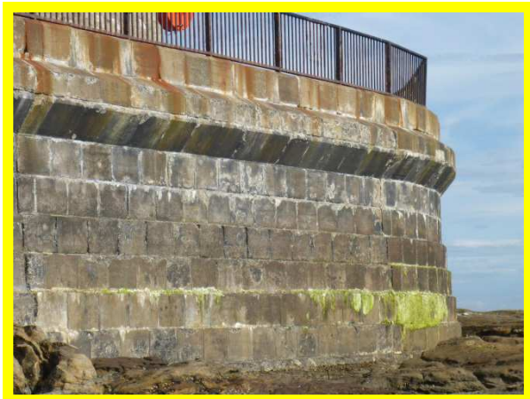
Brown's Bay northern sea wall in generally fair condition (/4601C10) (/4601C10)
