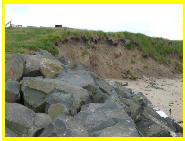
Erosion adjacent to rock revetment by St Mary's Island causeway (/4401C24)
