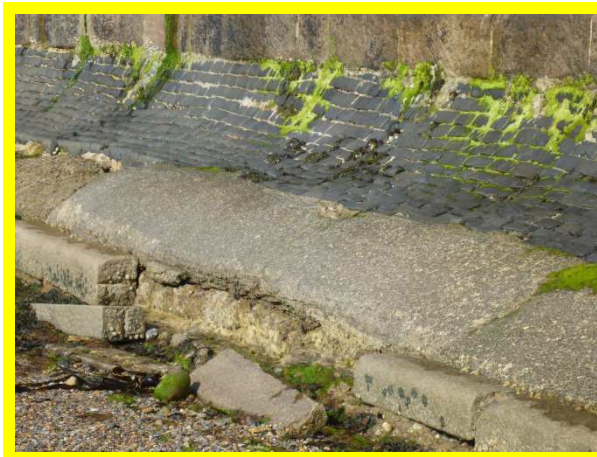
Final section of sea wall in generally fair condition, but with some defects at the toe requiring remedial attention (/4701C06)
