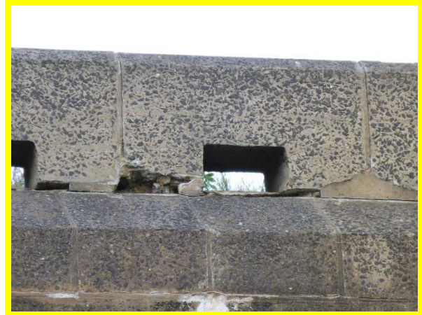
Cracked coping unit (/4501C07)
