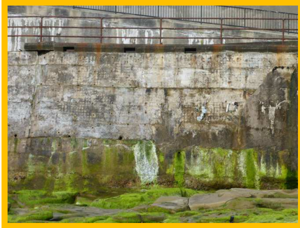
Loss of render and exposed reinforcement mesh (/4601C03)
