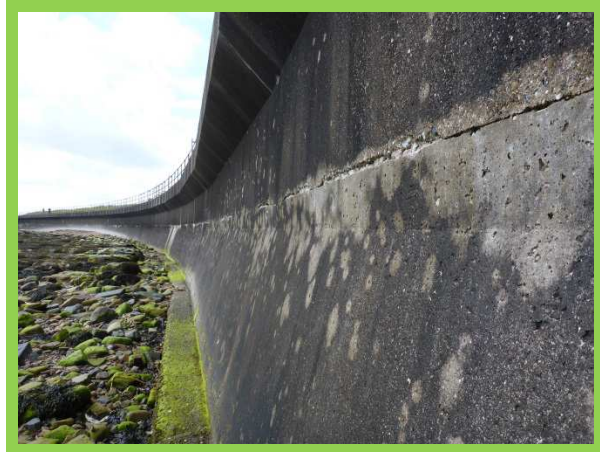
Trinity Road seawall in good overall condition, note the construction joints (/4501C04)
