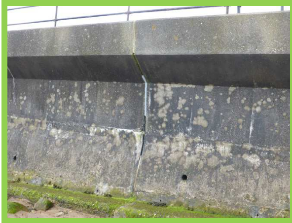
Trinity Road seawall in good overall condition, but with some minor maintenance required (/4501C04)
